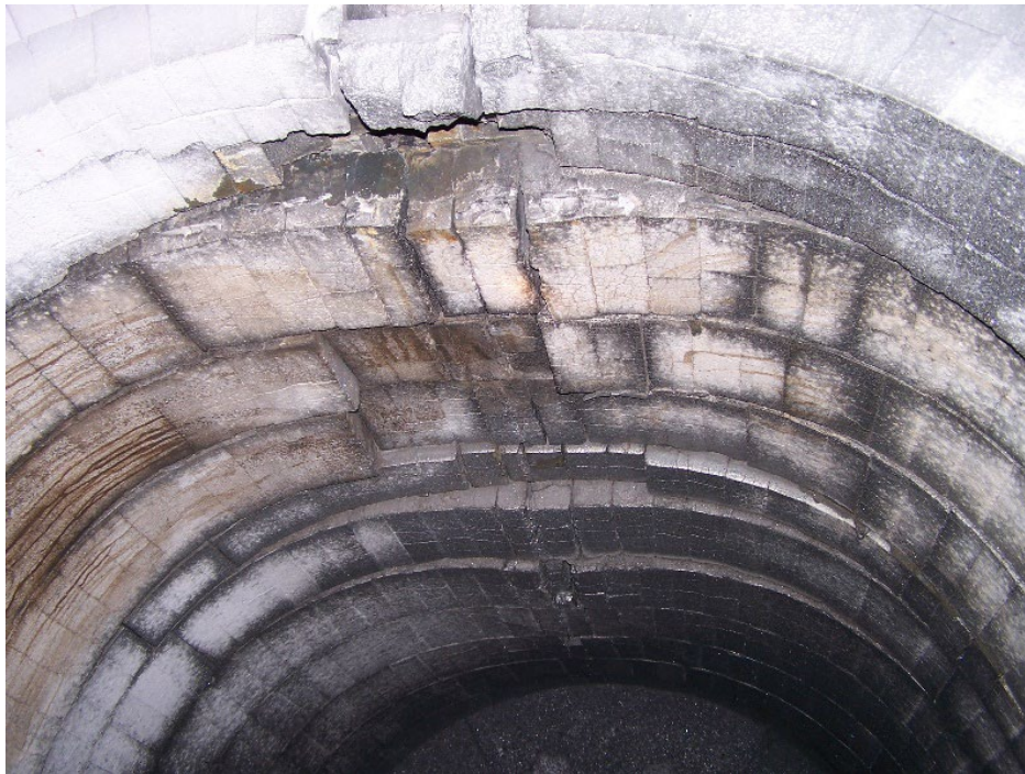
Figure 1. Damaged furnace refractory, likely caused by high temperatures.
