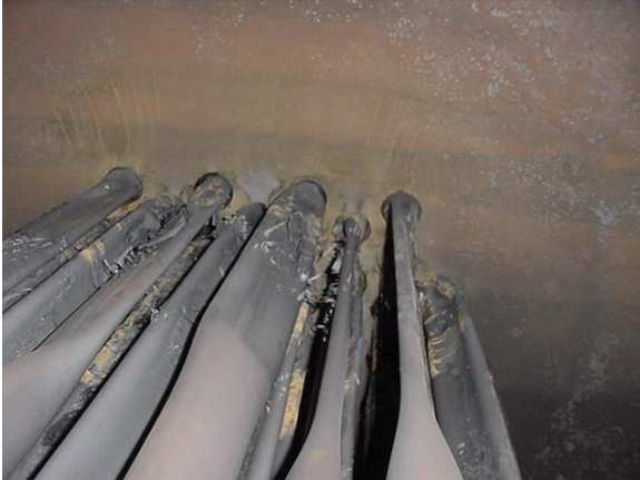
WHB Failure from Overheated Tubes
